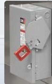
Fused Disconnect with Lock Out / Tag Out System
